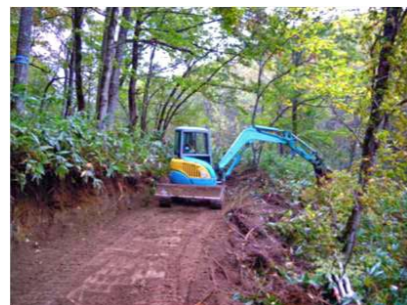
Construction of a “forestry operation road” for forestry machinery such as forwarders (National forest in Shibetsu-shi) [Kamikawa Hokubu District Forest Office]
